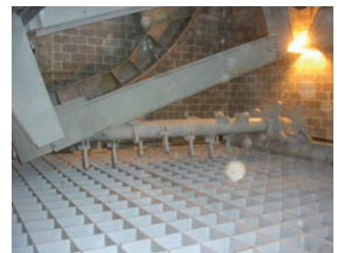
Hammermill installed and ready for use.
